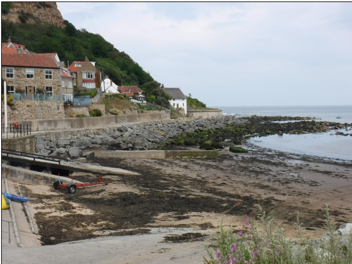
Figure 2.1. Location of new granite rock armour at the foot of the seawall, note the green (colonised) natural boulders which have been placed in front of the granite rock (July 2019).
